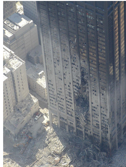
(Fig. 6) An example of girder damage to The Bankers Trust Building. It stood much closer to the South Tower than WTC 7 did to the North Tower, but it wasn't "scooped out" by debris.
